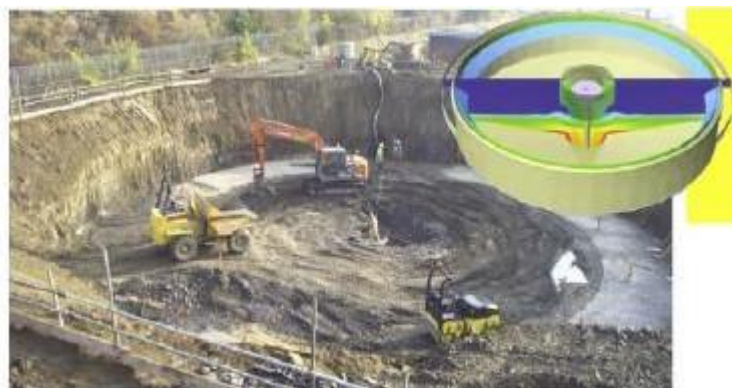
Figure 1.9 Example of CFD application to the construction of a new tank at a water treatment plant. The top right-hand corner of the figure describes the CFD simulation of the water tank that will be installed within the excavated construction site
